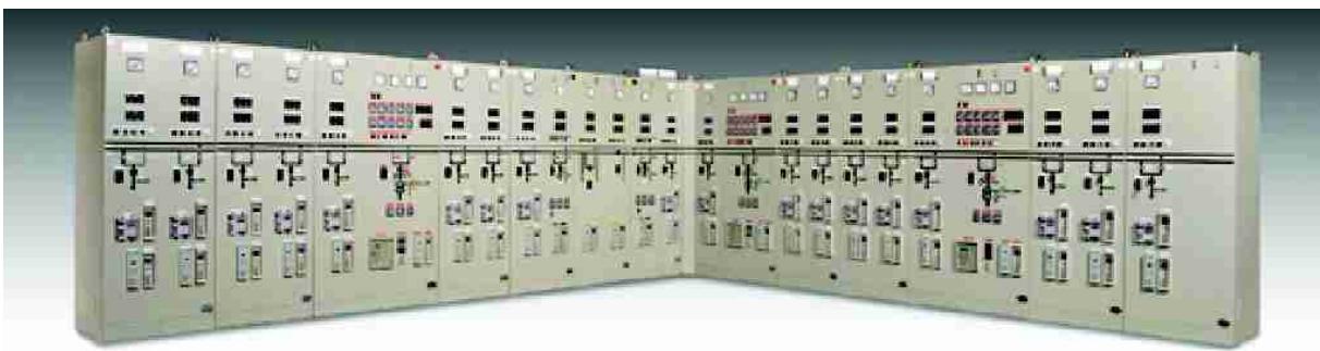
11 kV Remote Control and Protection Board In 'L' formation
