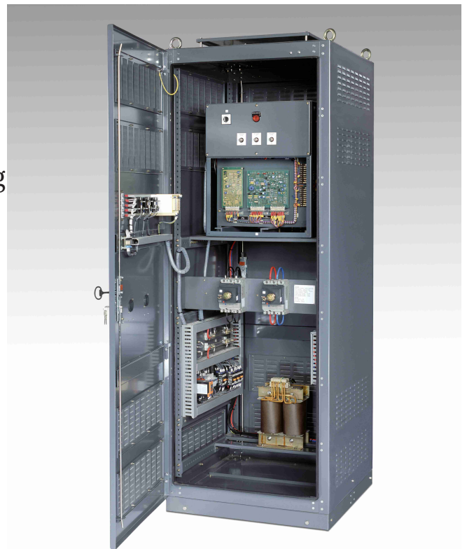
50VDC, 45A BATTERY CHARGER
